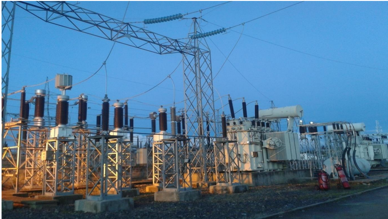
Figure 10 Debre Berhan Distribution Substation
