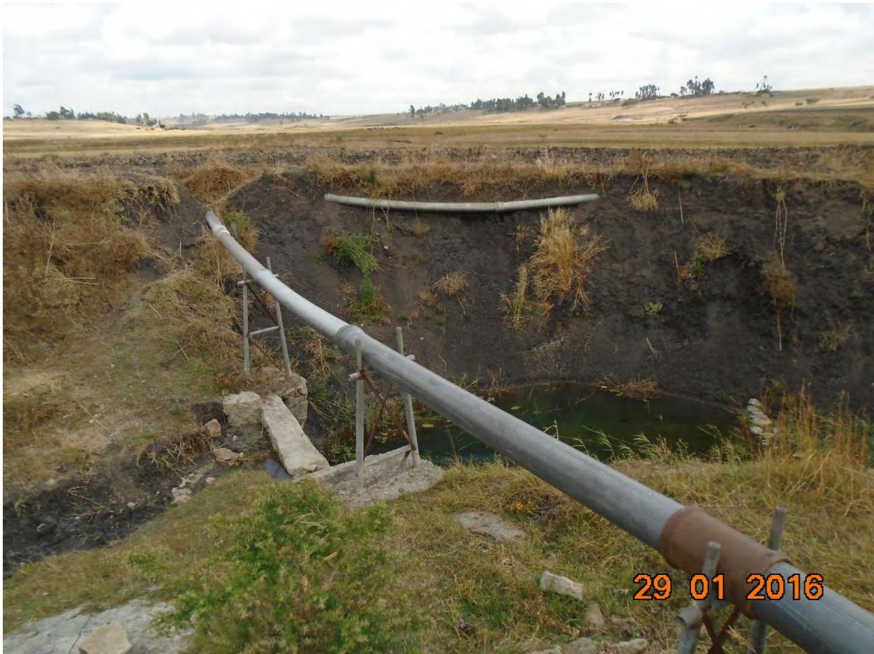
Figure 18: GFWS Project main line affected by gully
