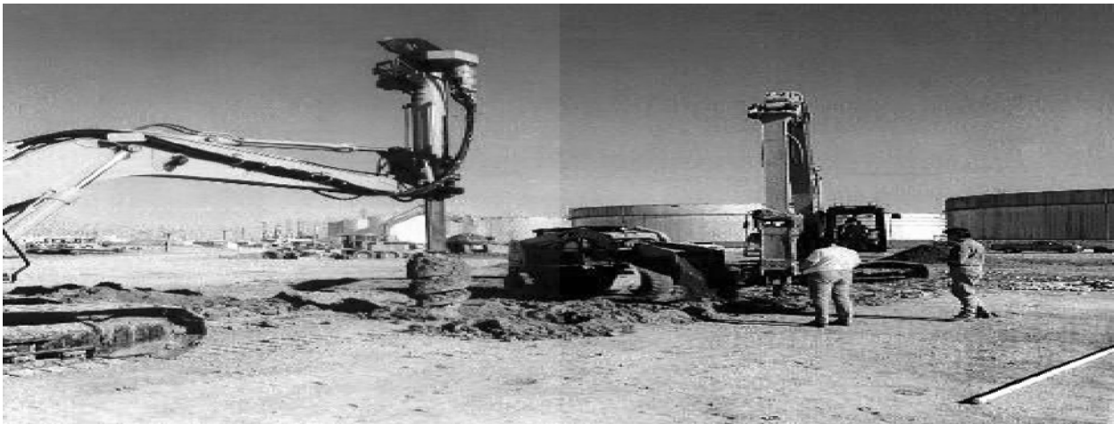
FIGURE 12.32 Installation of rammed aggregate piers, a type of stone column. (From Geopiers Foundation Co. With permission.).
