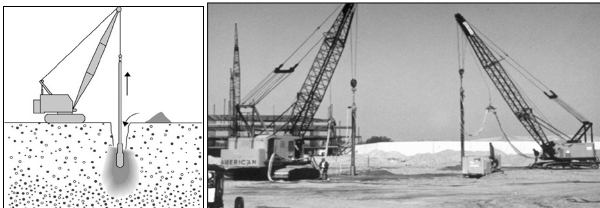
FIGURE 1.a Vibroflotation: (a) schematic, (b) field implementation. (From Hayward Baker Inc. With permission.)
