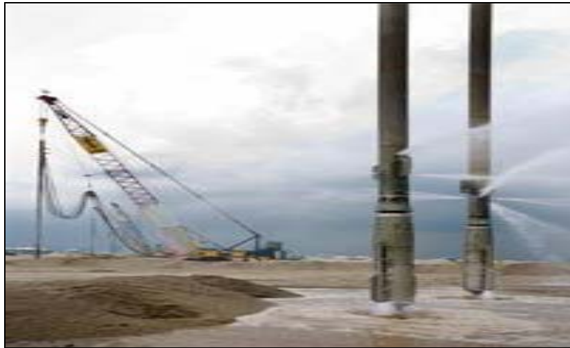
Figure 4. Twin vibro compaction rigs during the compaction works at the Universal Terminal
