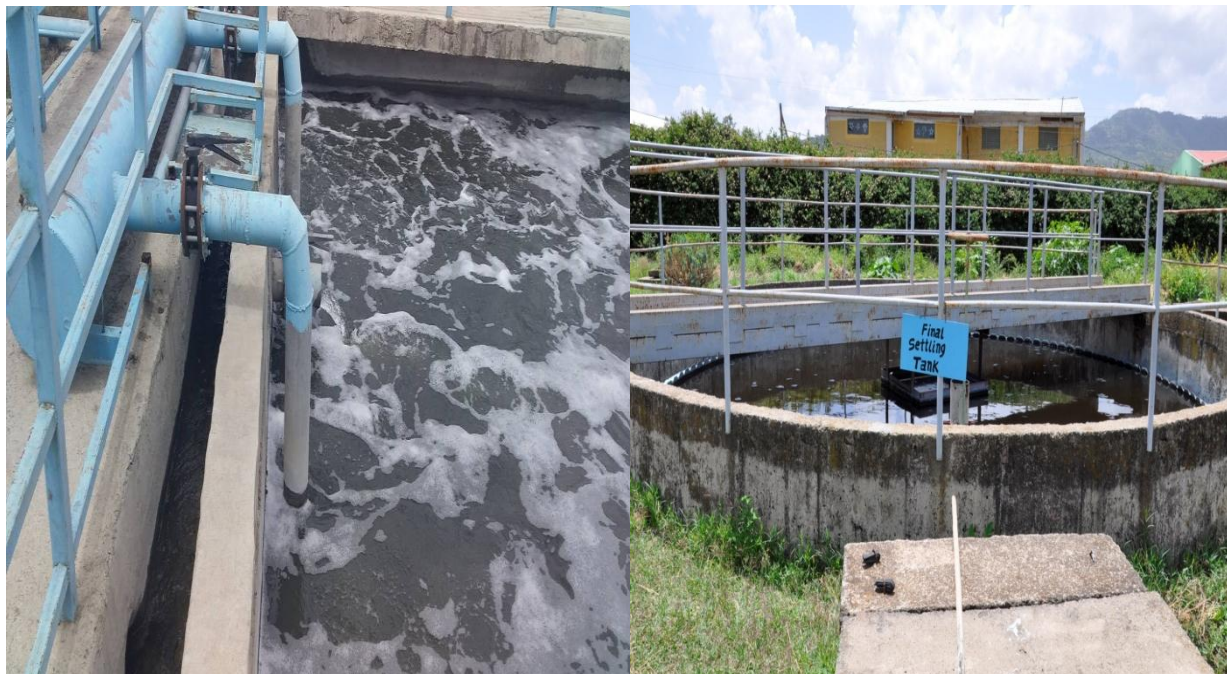
Figure 7. Secondary (biological) treatment and secondary clarifier/sedimentation tank in Kombolcha textile Sh. Co. (Self captured picture)
