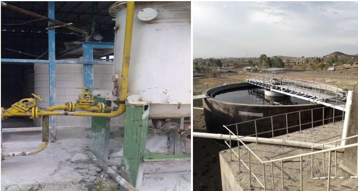
Figure 6: Primary treatment and primary sedimentation tank in MNS textile factory (Self captured picture)
