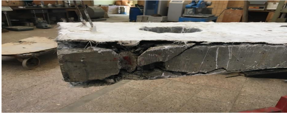
Figure 4-14 De-bonding of GFRP and crushing of concrete at 340.14KN
