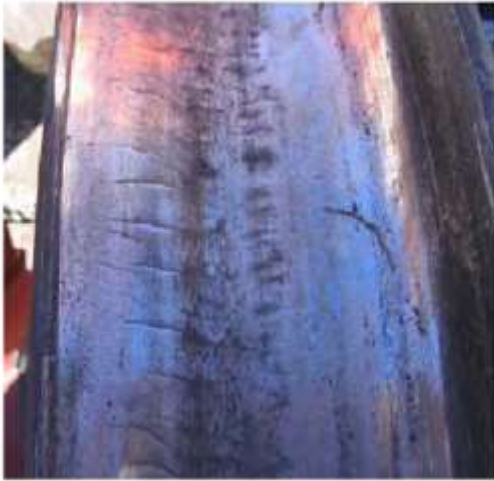
Figure 9: Rolling fatigue cracks on the tread [44]
