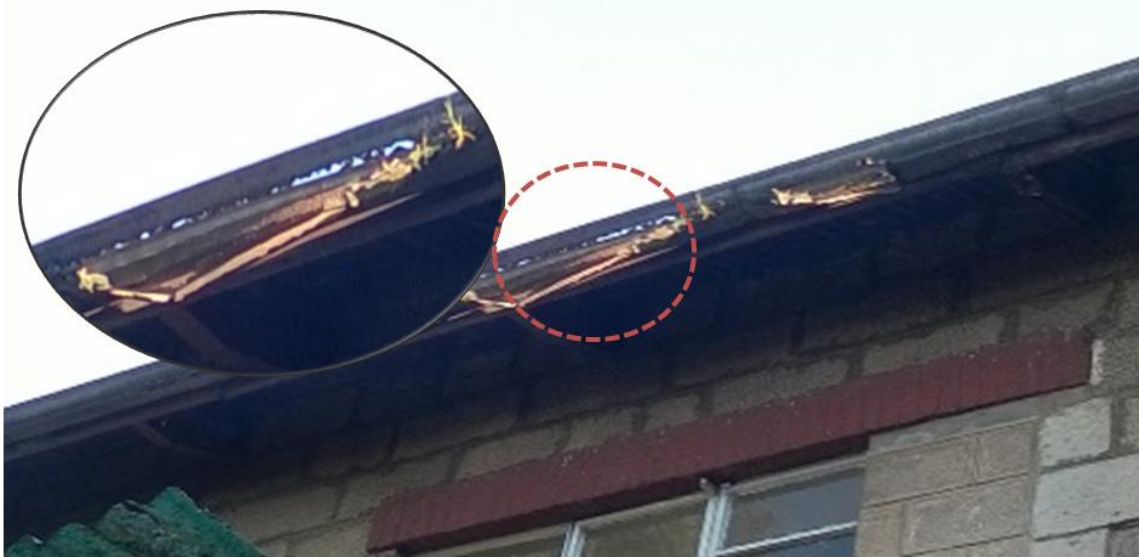
Figure 15: Trapezoidal gutter system at pathology building
