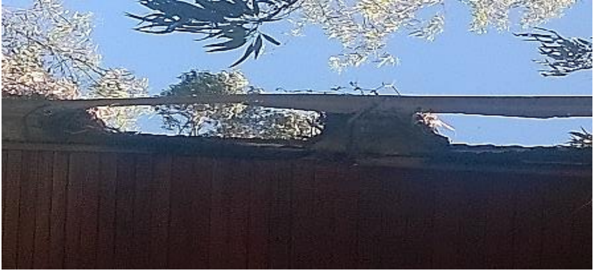
Figure 13: Trapezoidal gutter system on Animal House
