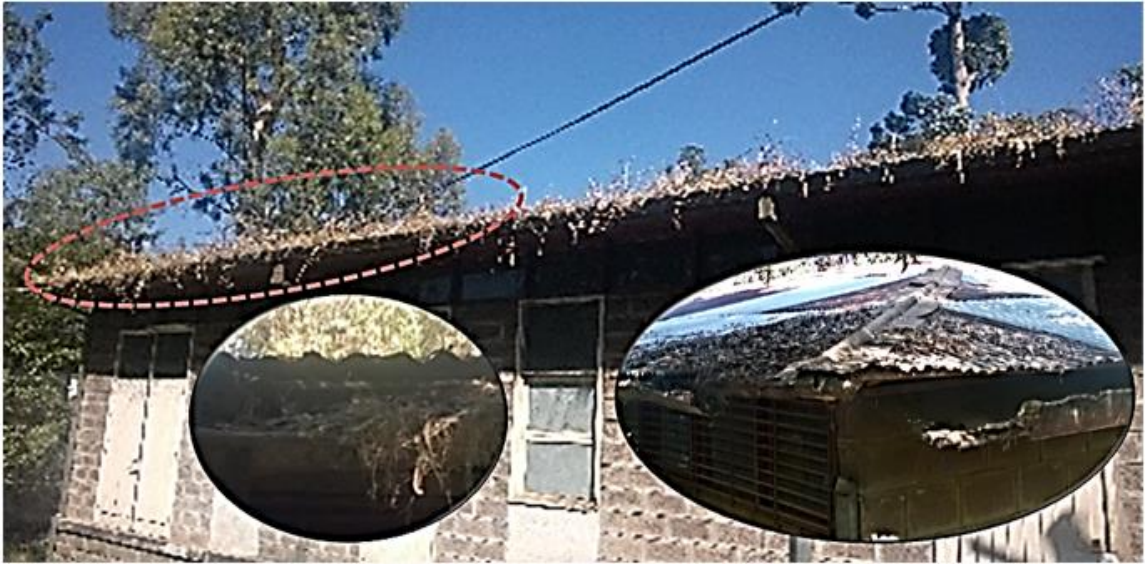
Figure 11: Trapezoidal gutter system on Animal House
