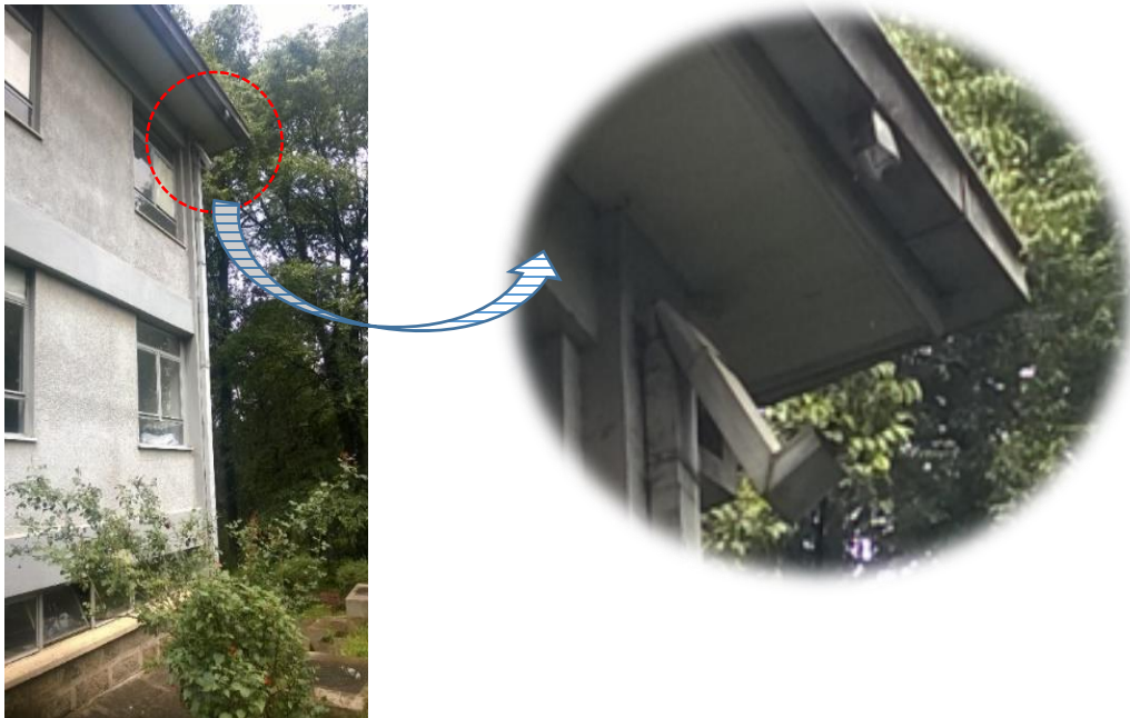
Figure 27: Dismantled downpipe system on urban buildings
