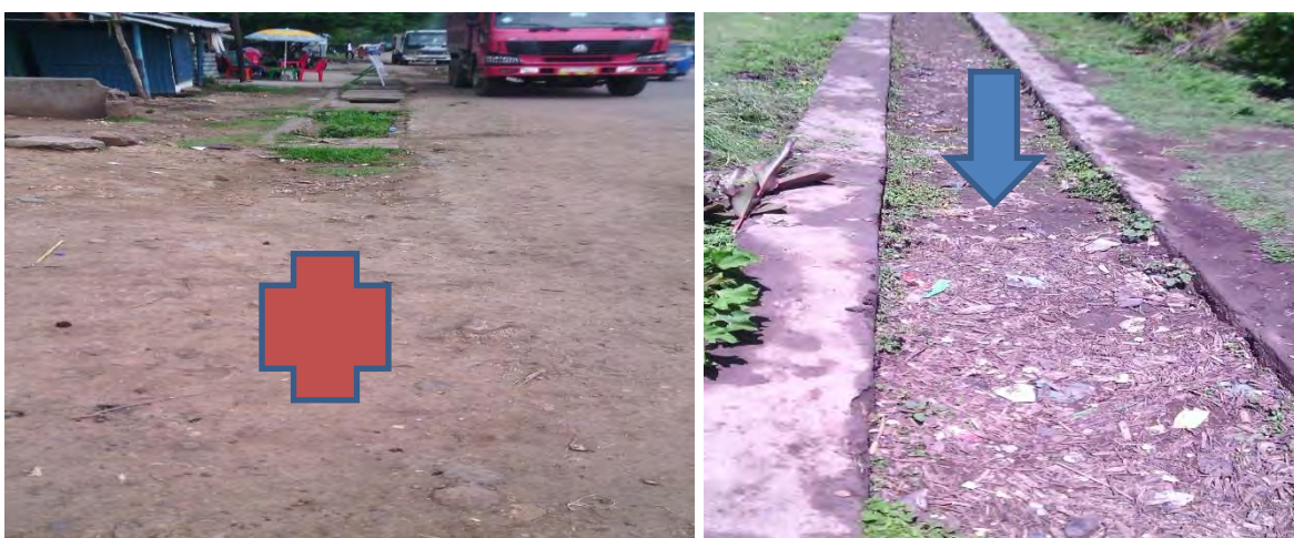
Figure 4.2 Crossing of access-road along with drainage and filled by sediment
