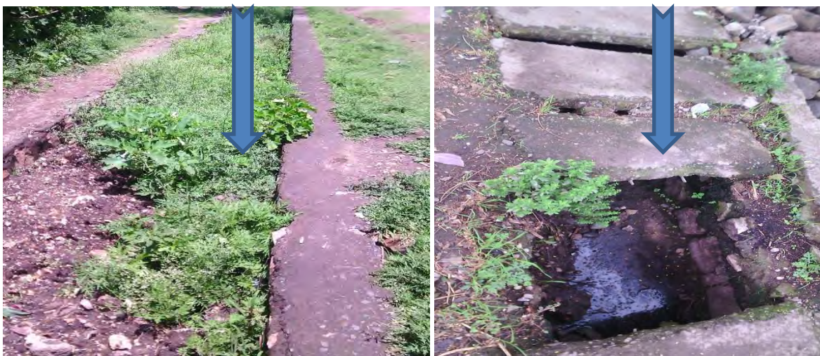
Figure 4.4 Half open and half close drainage system silted and grassed
