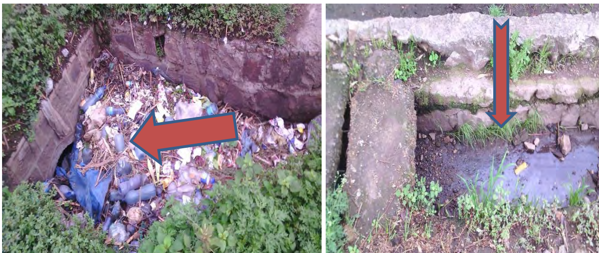
Figure 4.1 Drainage facility filled by rubbish materials and Small size of ditch along main road
