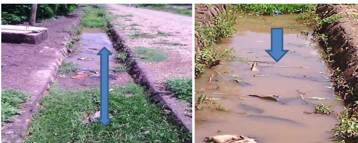
Figure 4.3 Open drainage system with no outlet and improper slope
