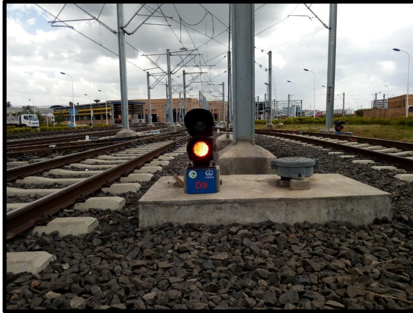
Figure 4. 11: Signal light at AALRT Kality Depot
