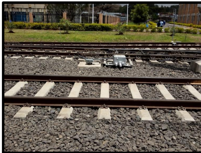
Figure 4. 10: Point machine at AALRT Kaliti Depot
