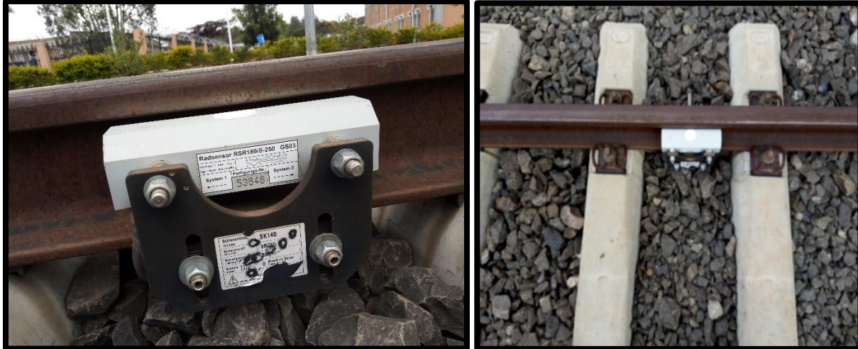
Figure 4. 7: Axle counter on the track
