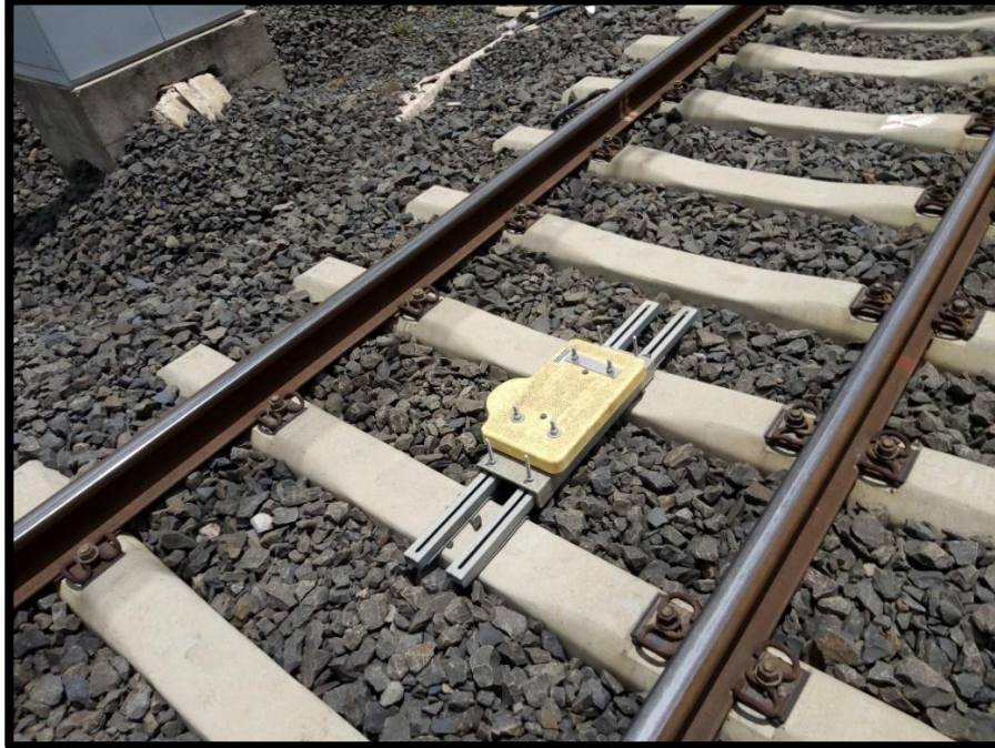
Figure 4. 12: Euro Balise at AALRT Kality Depot
