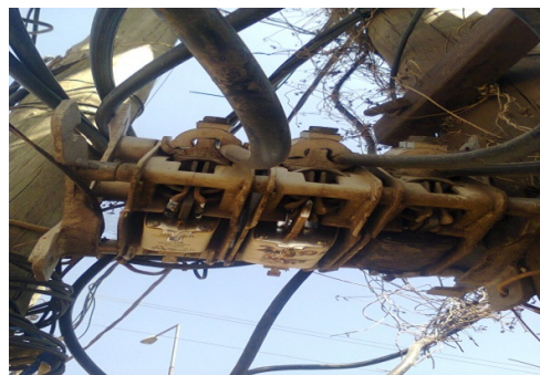
Figure 4.3 Sample photo taken for dust accumulation on switch gear [By Author]
