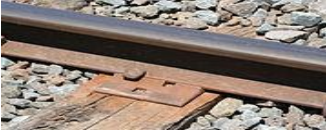
Figure1.7. Rail spike with baseplate above the tie
