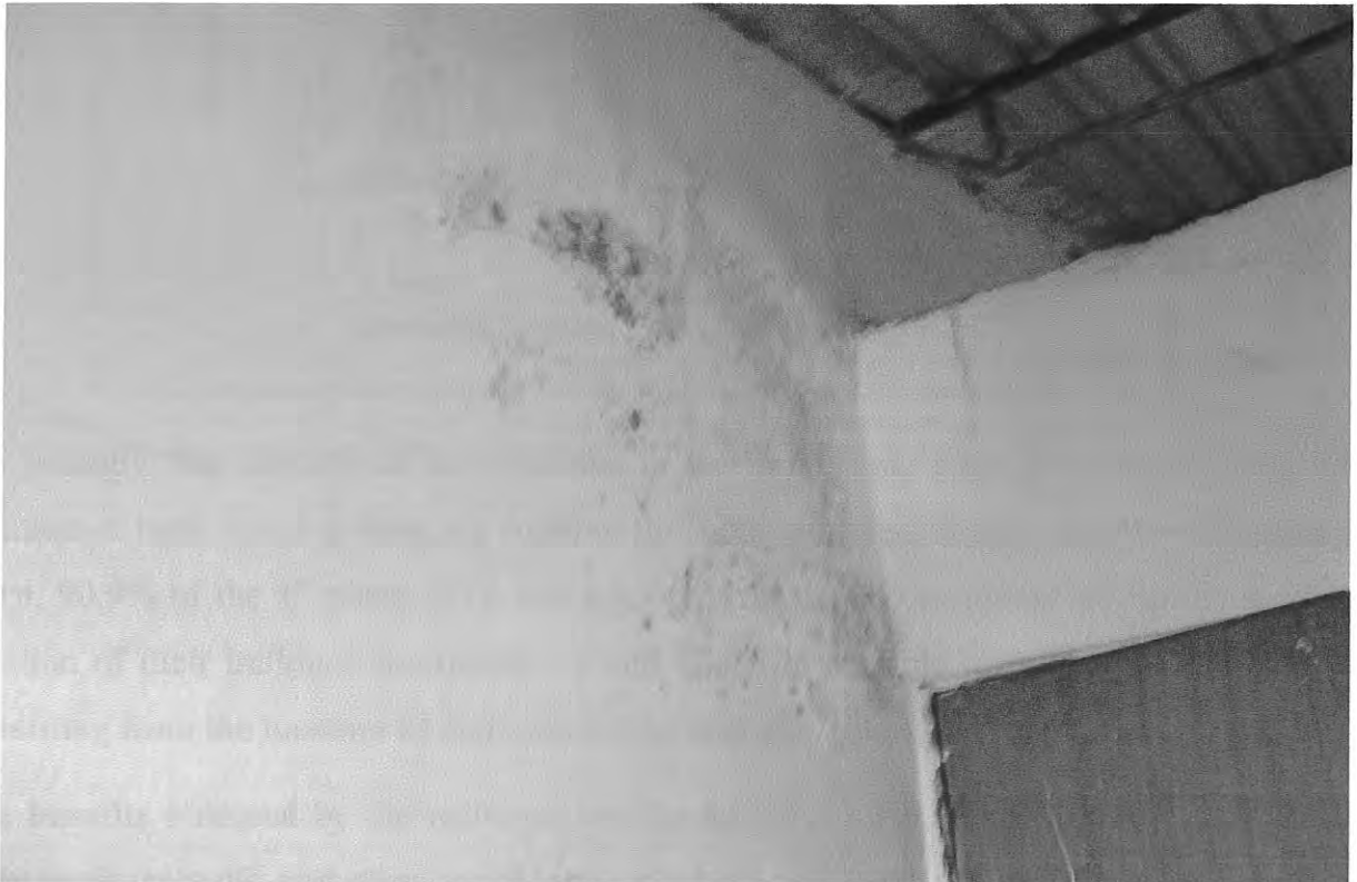
Fig. 20 Photo showing leakage problem on a wall structure on the Balcha site of the GTZ.
