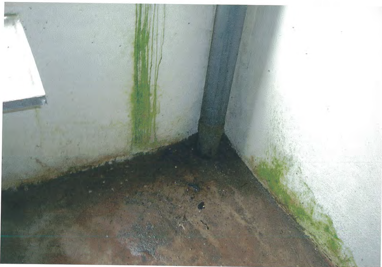
Fig. 18 Photo showing leakage problem of sanitary installation in the Balcha site of GTZ.
