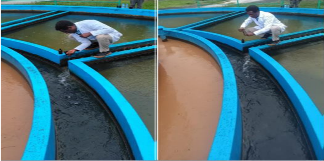
Geferesa Treatment Plant 1
