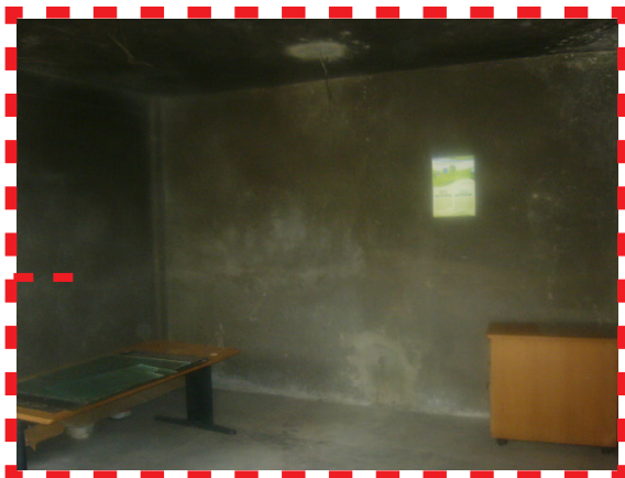
Fig. 8.11 The Unit owners association started to use office as recently as February 2016.
