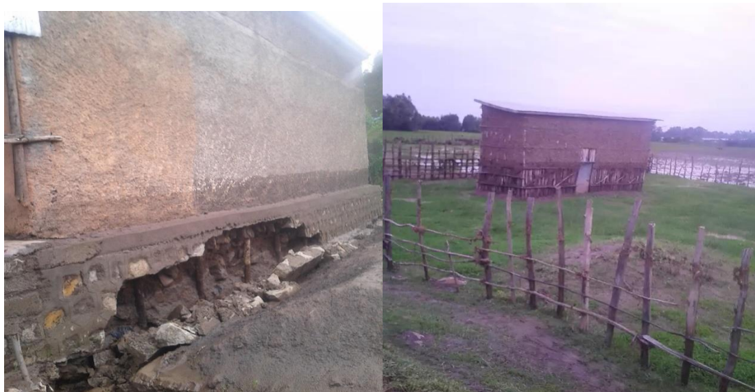
Figure 3.29: Building damage during a flood event
