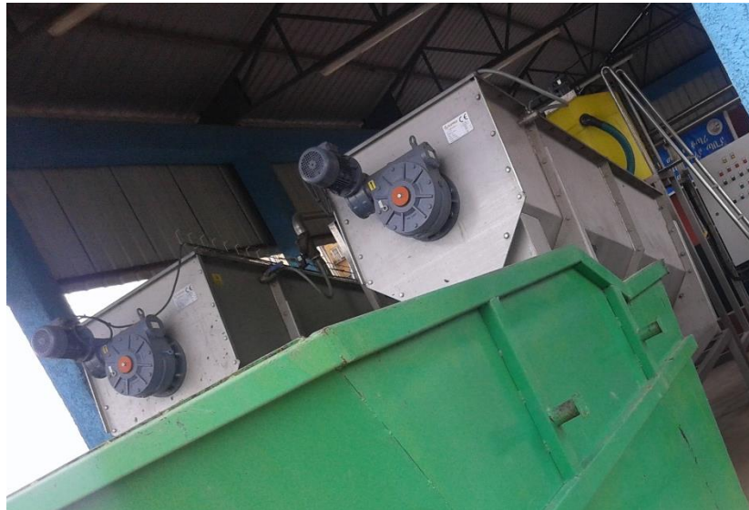
Figure 3-3 Decanter centrifuges for dewatering sludge
