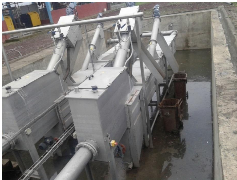
Figure 3-1 Combined unit with automatic screening and grit removal
