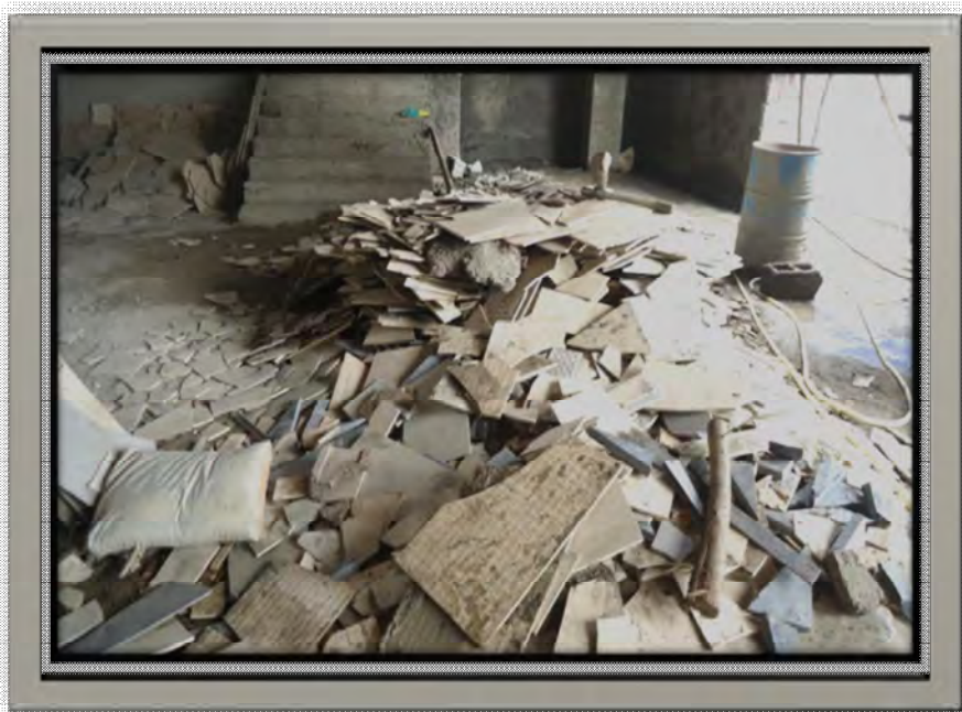
Figure 1 Ceramic tiles wastage in the construction site.
