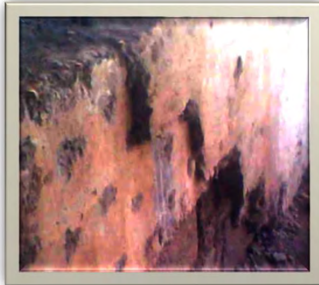
Figure 2 This Figure poor work man ship that cuase bulged out beam & over sized thinkness of plastering.
