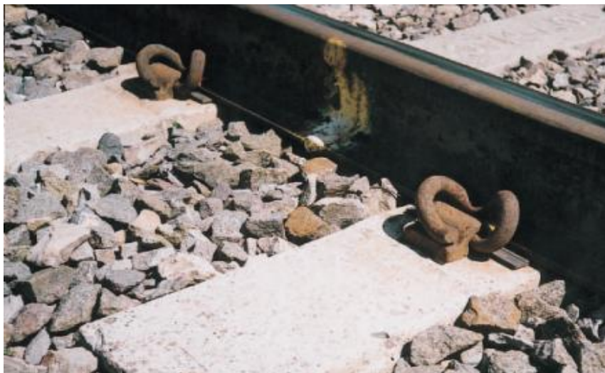
Figure 2-20 Rail ballast crushed stone aggregate on track
