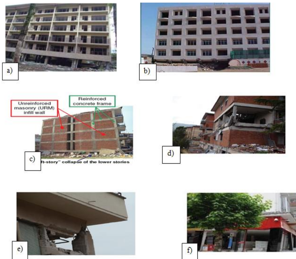
Figure 2.1 Masonry infill-related damage in recent earthquake
