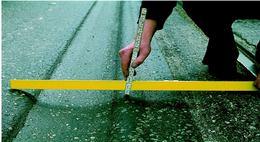
Figure 2-6 Rutting caused mainly by studded tire wear (Rabbira Garba, 2002)
