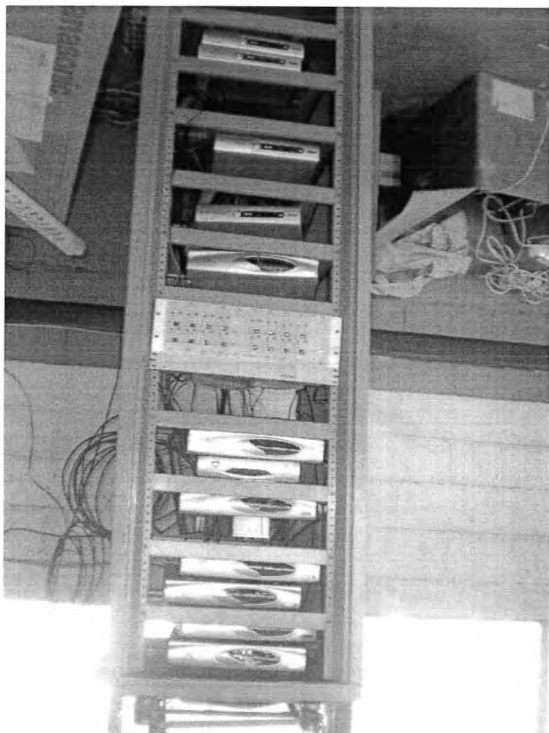
Figure 2 Transmission controller at Minilik II Secondary school
