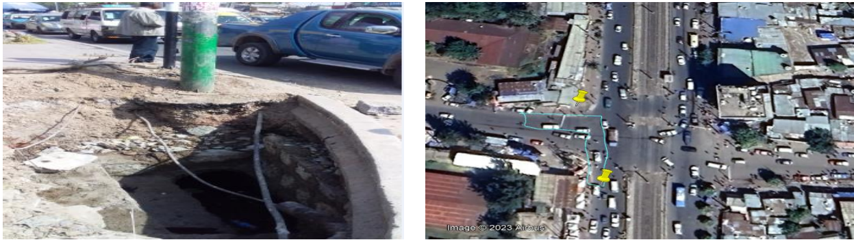
(d) Exposed and nearly missing utility strike
