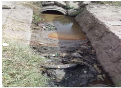
(a) Ditch blocked by solid wastes
