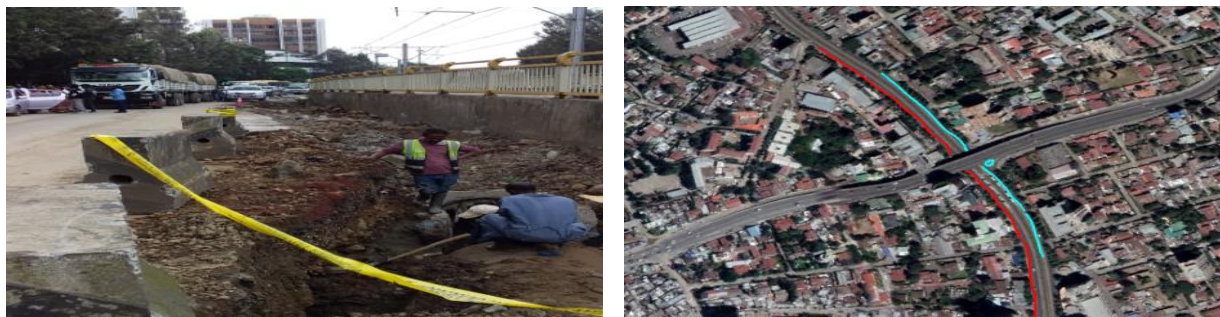
(d) Traffic congestion due to narrowed roadway segment under repair work (e) Google Earth location of excavation sites
