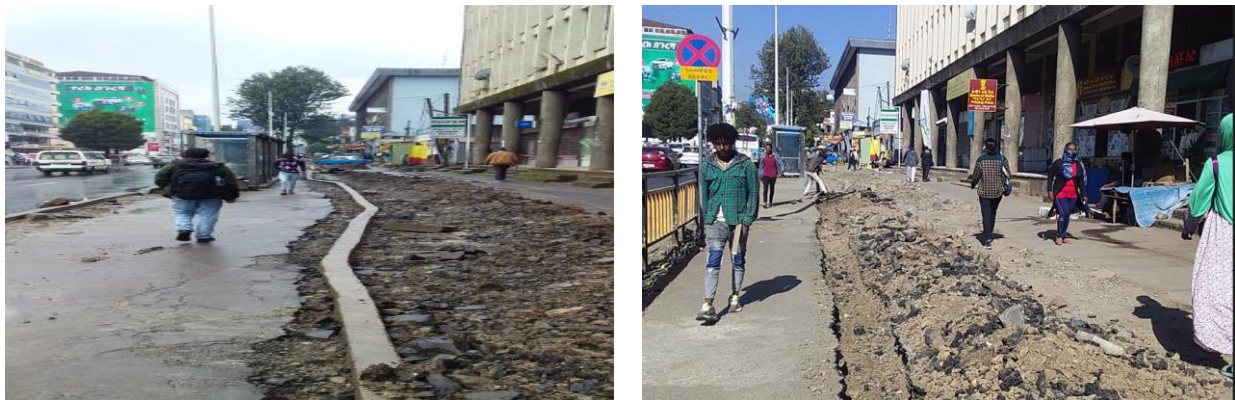
(d) Constructed curb stone and poorly reinstated excavated walkway (e) Repeated trenching and inconvenience to users
