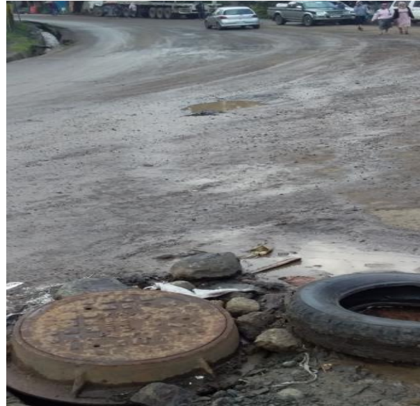
(b) Clogged/blocked manhole with removed cover
