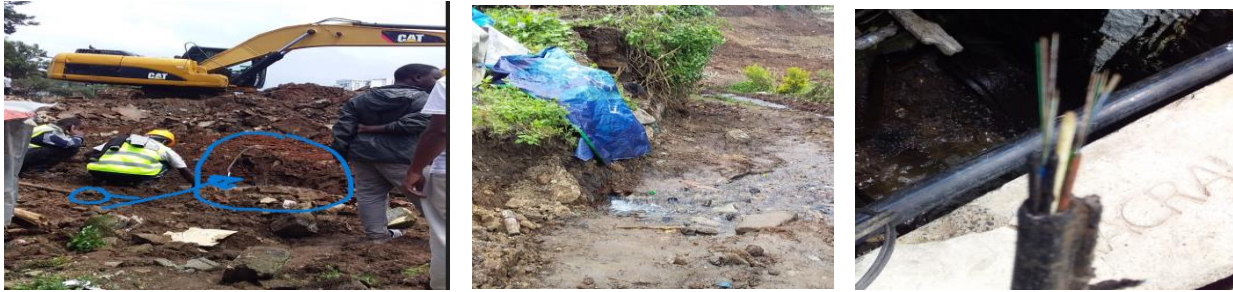
(a) Damaged invisible utility line during excavation (b) wastage of scarce water due to damaged pipe (c) damaged fibre optics
