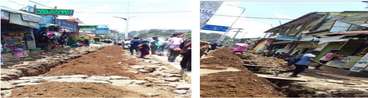
(d) Inconvenient travel and access to shopping centers (e) loss of customer and/or income to firms due to excavated trench Fig.4.18: Indirect economic impacts of repeated excavations to existing city infrastructure (captured by author on 25/9/2023)
