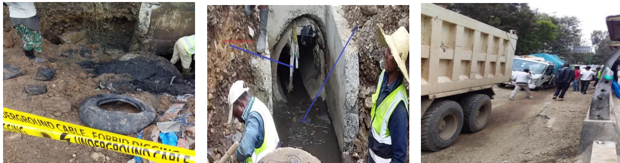
(a)Excavation & removal of solid waste from drainage line (b) Repairing drainage line (c) About overtuning traction trapped loaded vehicle
