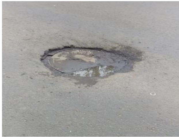
(e) Poorly constructed manhole
