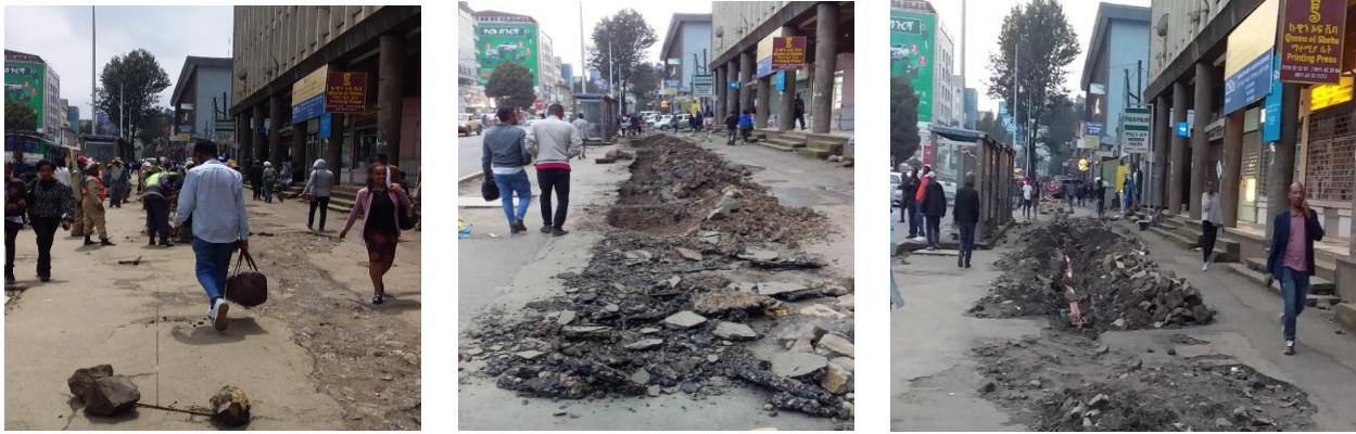
(a) Previously excavated walkway (b) trenching twice within week (c) poor installation and reinstating of the trench
