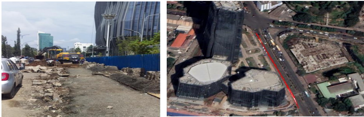
(d) Pedestrians & motorists sharing common roadway at excavated section (e) Google earth image location of the excavation site
