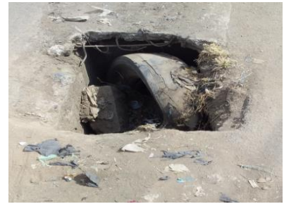
(c) Clogged & damaged drainage line
