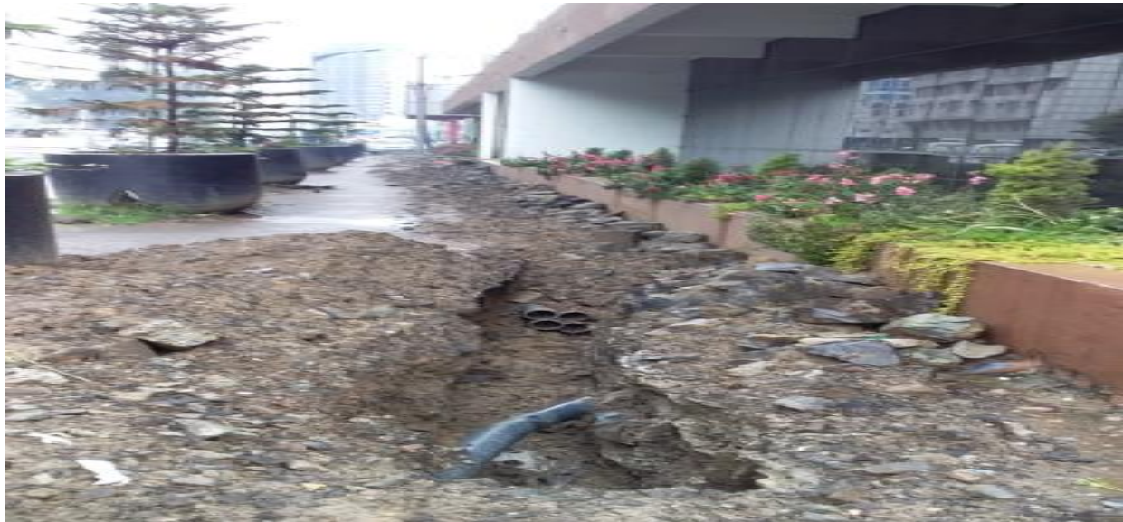
(c) Exposed and damaged utility lines
