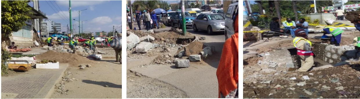
(a) Construction material and workers at repairing work (b) excavated pit and Vehicles versus pedestrian (c) repairing work
