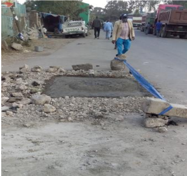
(a) Repeatedly repaired manhole & barriers to users
