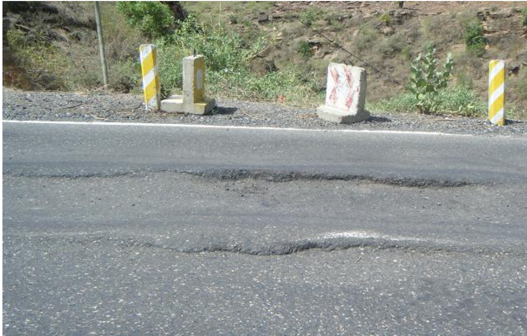
Figure 1.1 Condition of Goha Tsion – Dejen Road
