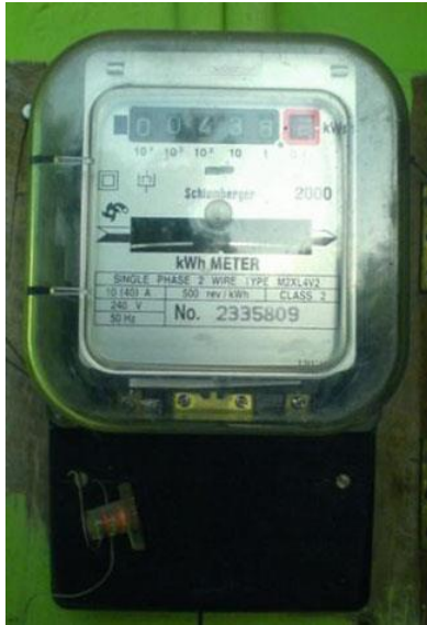
Figure 2-1A single phase electromechanical meter [8]
