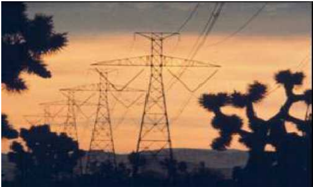
Figure 2.1: \pm 5 HVDC transmission line [17].
