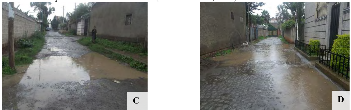
Figure 6. 28 Waterlogged local streets in Mekerbetoch area Source: Fieldwork (2016)
