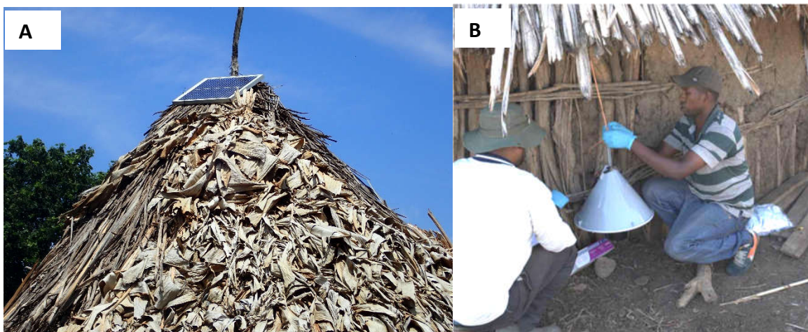
Figure 5.2. Solar panel installed on the roof of a house (A) and installation of the odour-baited trap (B). Picture Credit (A: Yared Debebe and B: Prof. Rickard Ignell).
