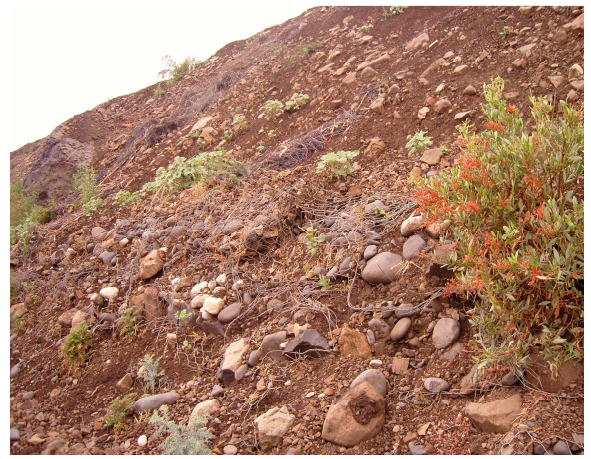
Damage on Gabion wall
