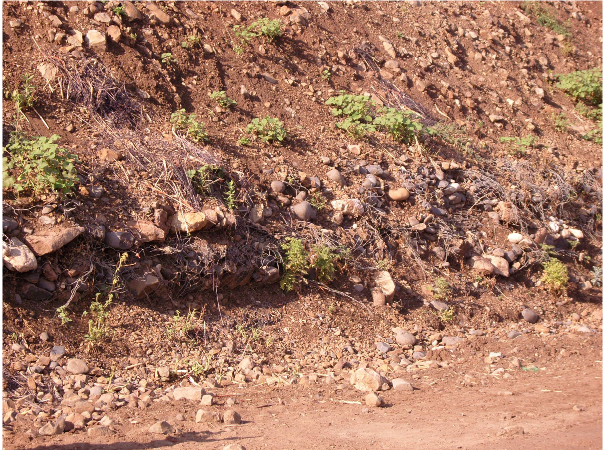
Fig. 6.4 Damage on the Gabion wall
