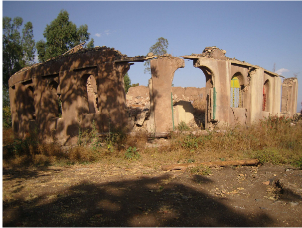
Damage on the old church
