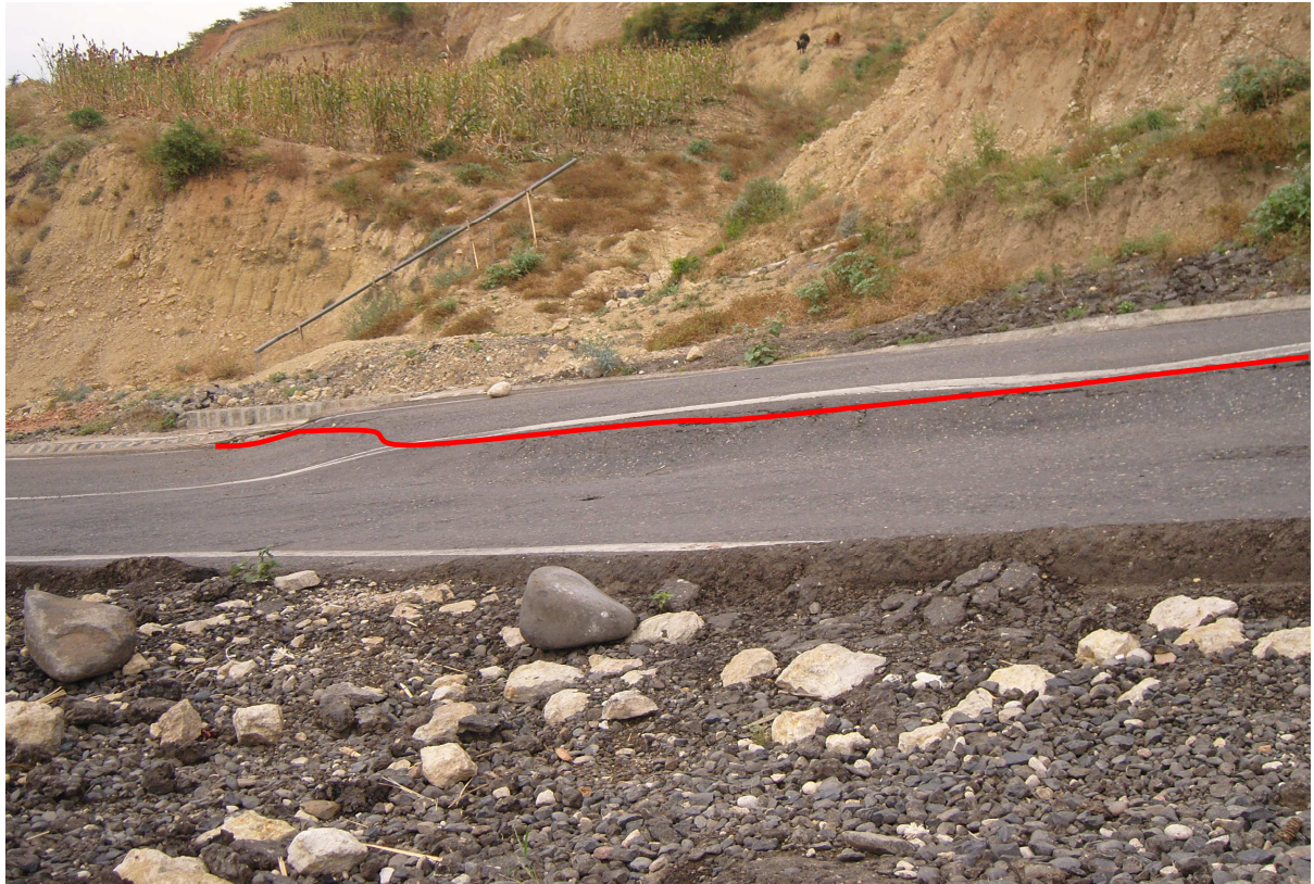
Fig.4.9 Photo showing tension crack on the road
