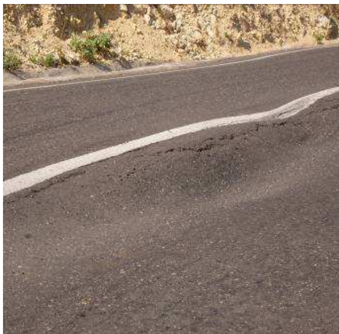
a. Damage on the main road
