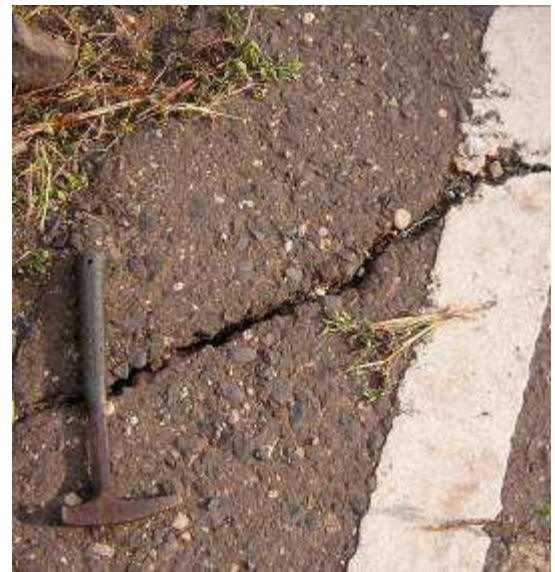
b. Tension crack developed on the road
