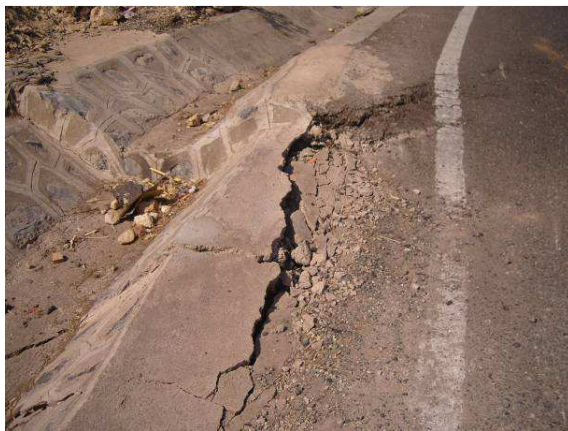
Damage on the road
