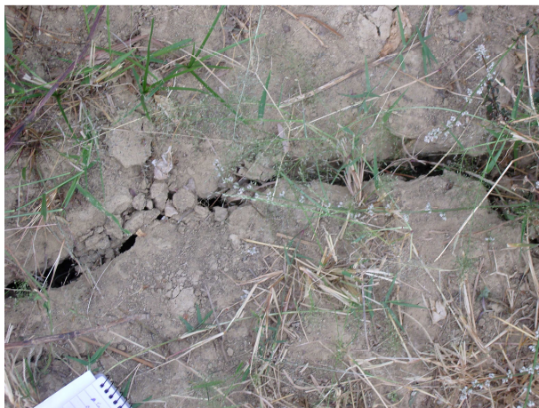
Tension crack on soil mass
