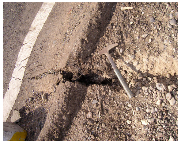
Tension crack cutting the road
