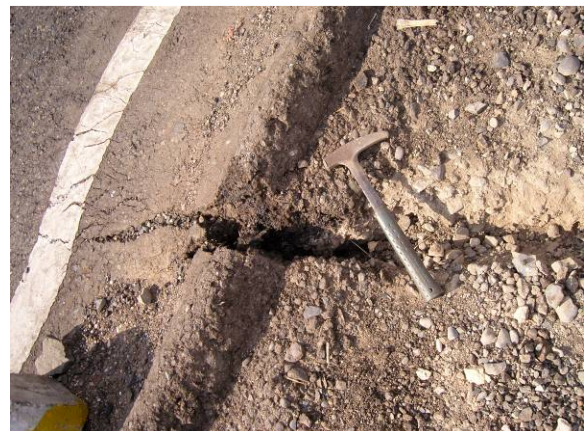
Tension Crack on the road
