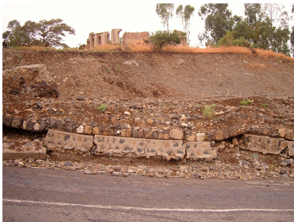
Massive slide on the road
