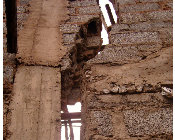
Damage on the church under construction
