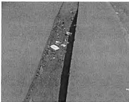
Figure 4.6 Picture showing Un maintained roads
