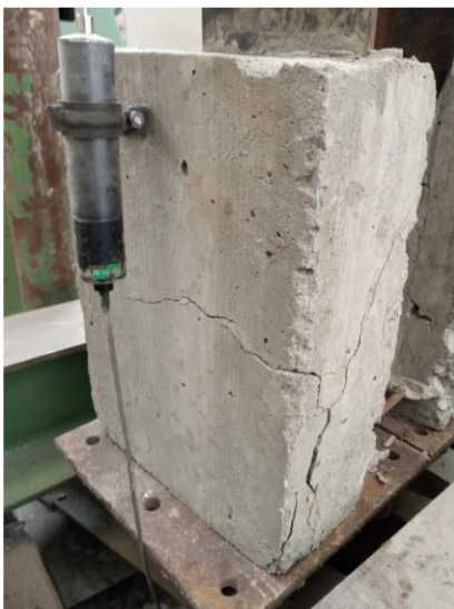
Fig 4.7): failure mode of Specimen S-C-2
