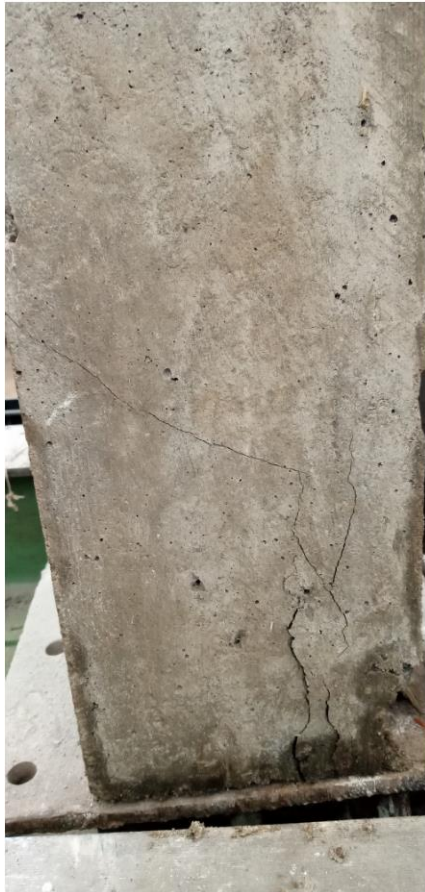
Fig 4.10): failure mode of Specimen S-D-5
