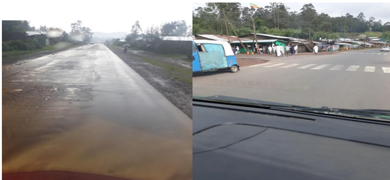
Figure 4.28: Lack of Pedestrian Walkway, Routine Maintenance and Traffic Sign at Intersection
