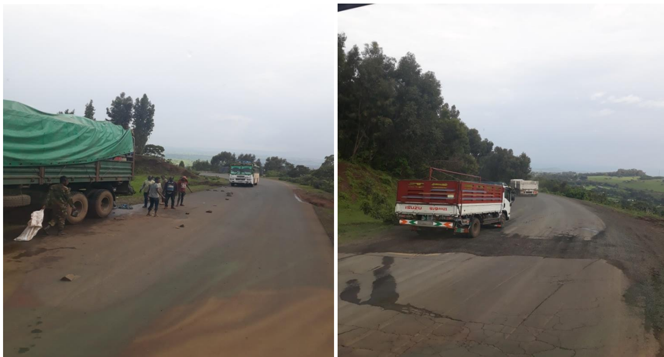
Figure 4.22: Photo of Invisible Pedestrian Crossing, Lane Markings and Lack of Routine Maintenance
