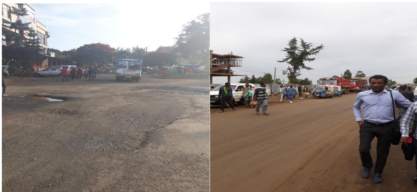
Figure 4.24: Improper Drainages, Lack of pedestrian walkways, routine Maintenance and Traffic Sign
