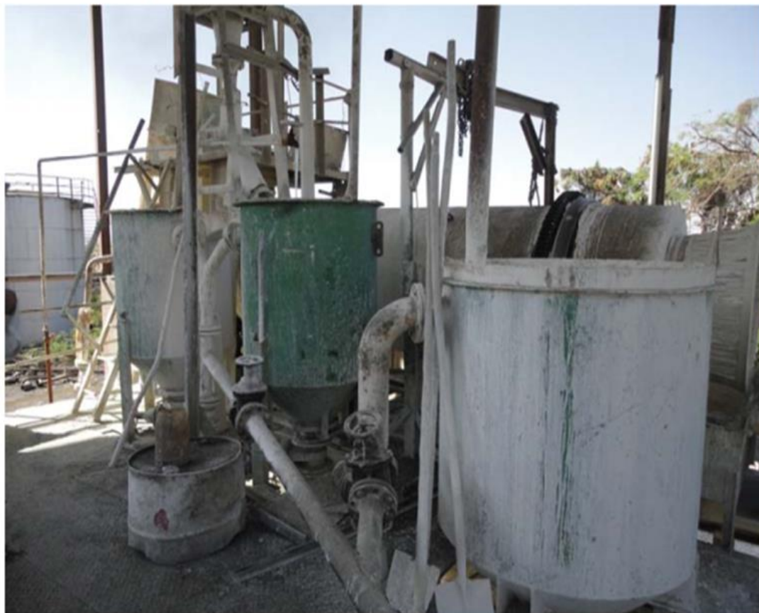
Figure 2.2: Milk of lime preparation plant of Metahara Sugar Factory
