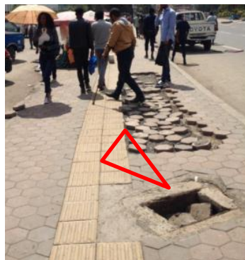
Figure 4.1-3: The street leveling problems impact
