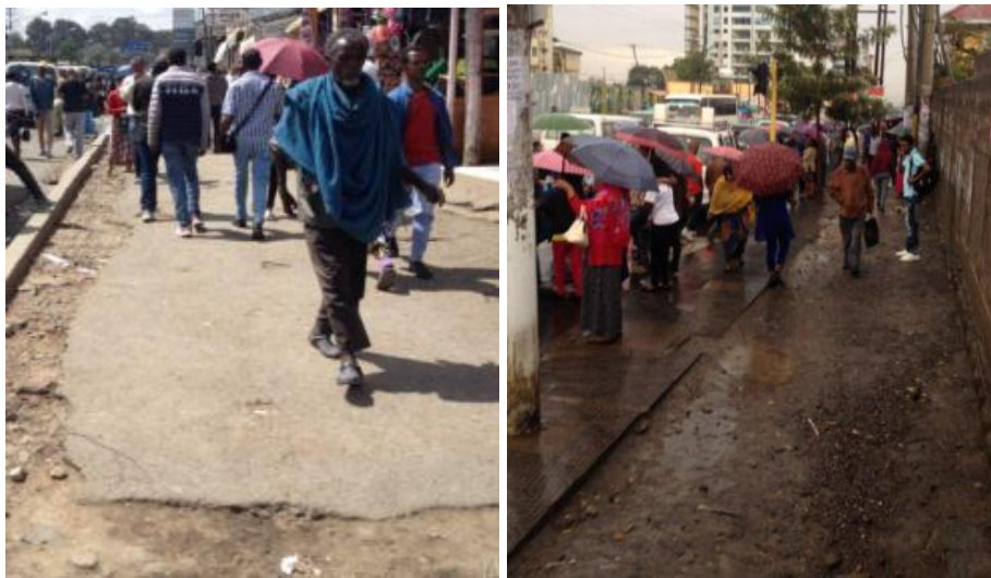
Figure 4.1.3-1: The problems due to weak design and construction of street
