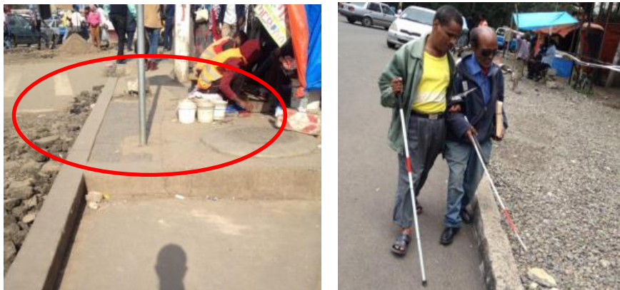
Figure 4.1-2 pedestrian walk way leveling problem and Street marketing impact
