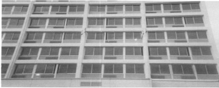
Figure 1: Shear- bond failure in 3rd story of Holiday Inn Hotel in Van Nus
