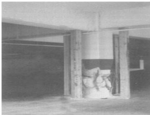
Figure 3: Shear - compression failure in column of cast-in -place garage in Sherman Oaks
