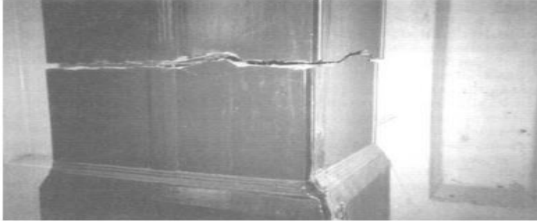
Figure 4: Column brittle failures observed in a steel Mega-truss at Ashiya-hama
