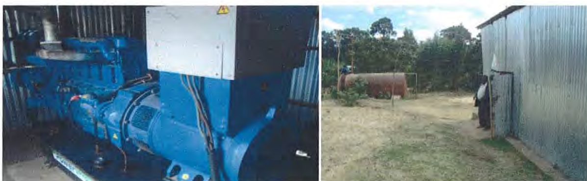
Figure 2: Generator at Gocho Bore hole
