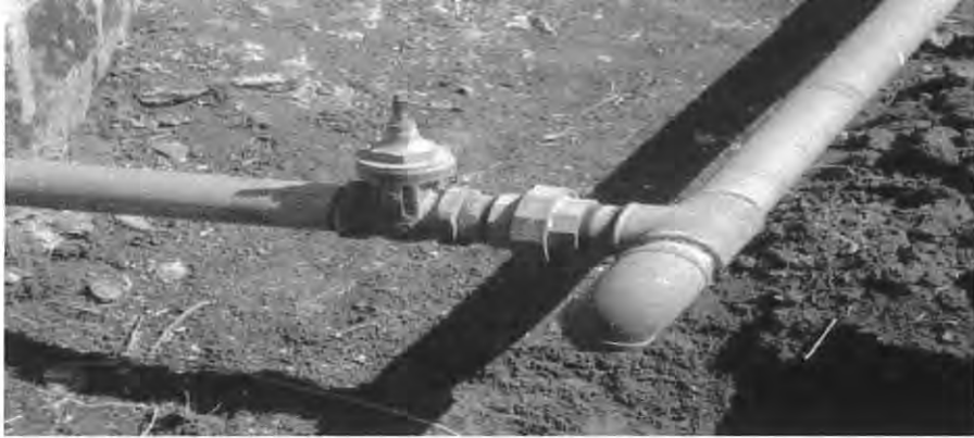
Figure 9: Pipe line at industrial college with no water at all
