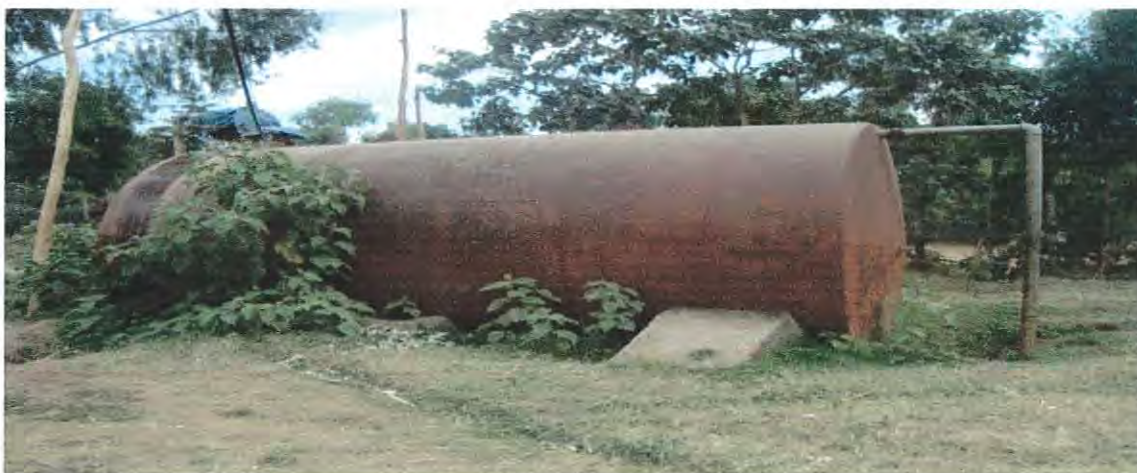
Figure 5: The steel wet well at booster station
