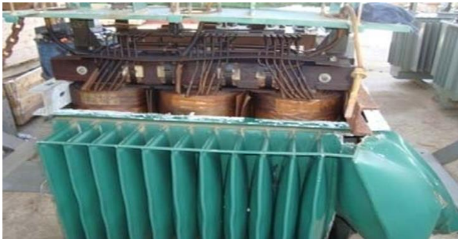
Figure 4.2: Burnet Transformer Picture due to overload
