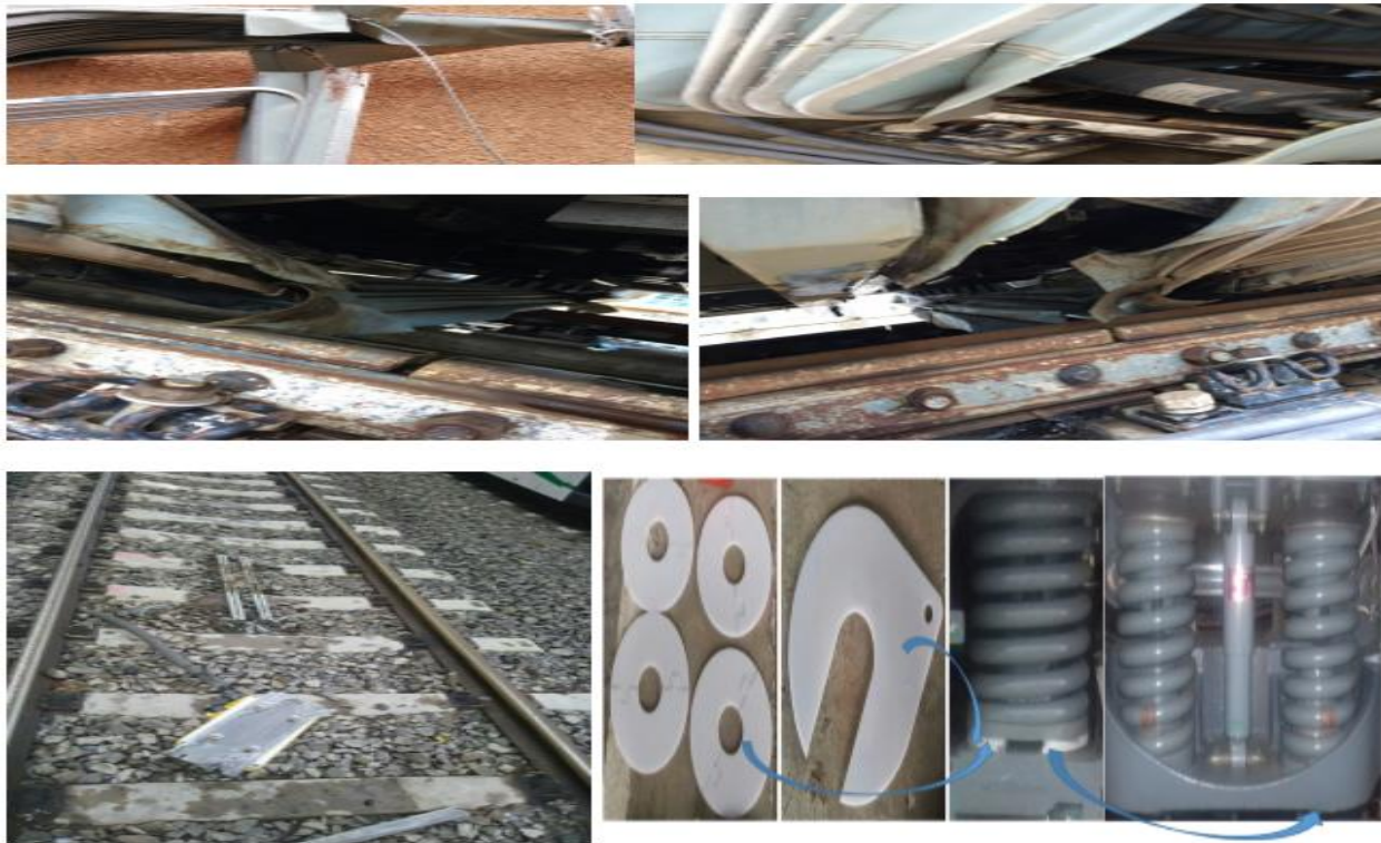
Figure 3. Vehicle body Lowering down and damaging of ballie from sleeper and damaging itself This figure collected from the problem faced vehicle. For the lower right on the figure is that, they used to minimize the lowering down problem.
