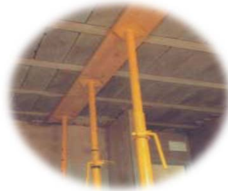
Figure 2.7 The soffit of a beam and block slab in place with support
