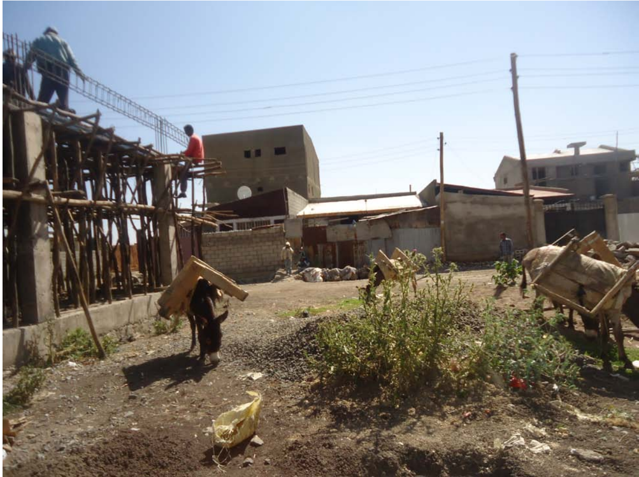
Photo 3: The picture of houses on the process of building in Ayat land replacement relocation site
