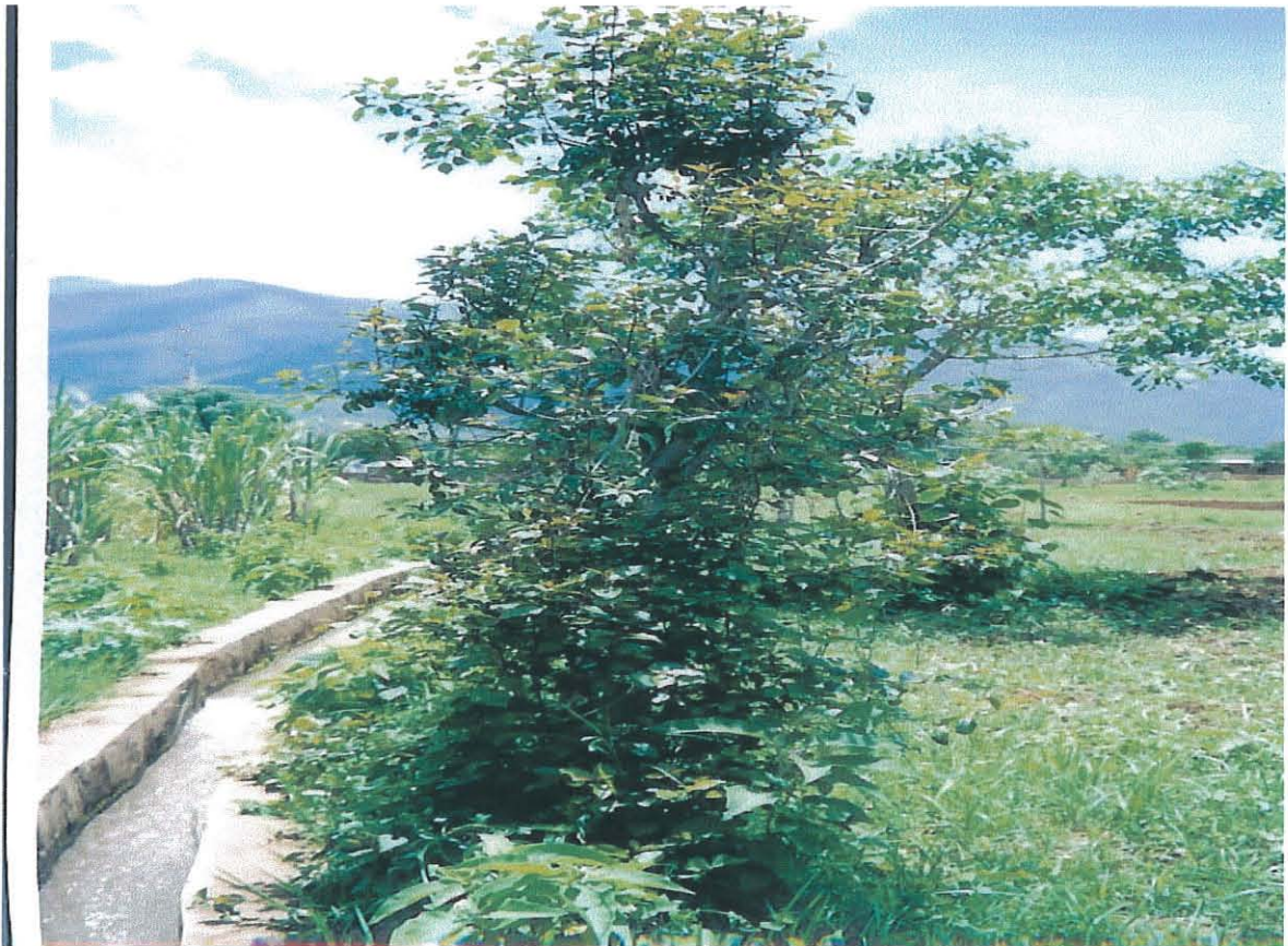
Photo 5.2: Cemented irrigation canal in Gamule crossing the irrigation plots
