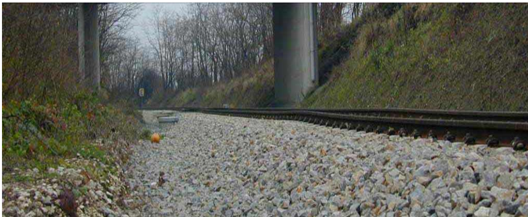
Figure 2.20: Bad track quality due to soft subgrade [Wenty, 2007]
