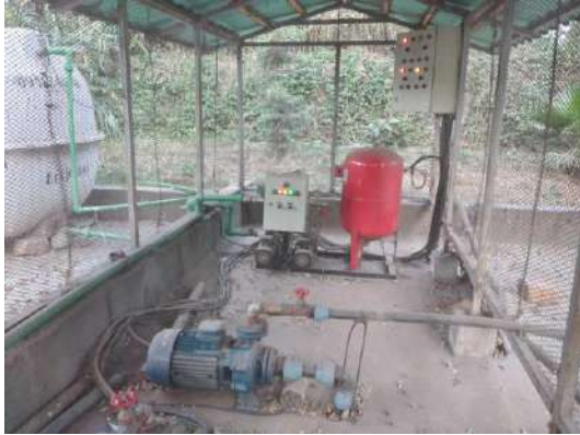
Figure 4.13: Water reserve with pumping system
