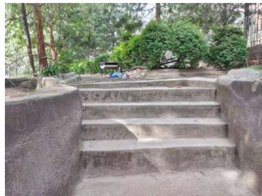
Figure 4.45: Uneven stair access to restroom
