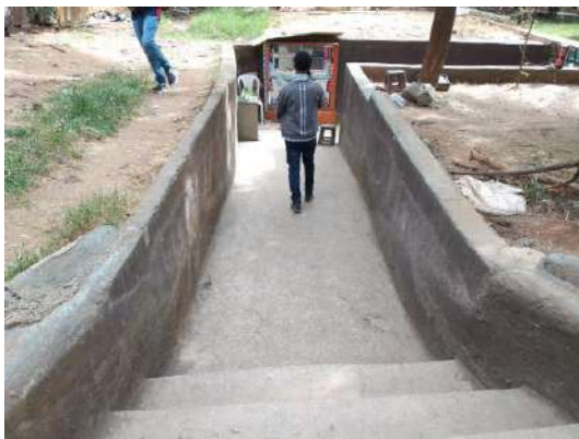
Figure 4.52: User unfriendly and uneven access to public toilet
