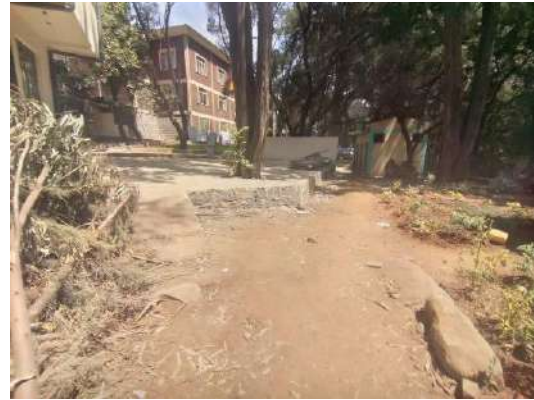
Figure 4.96: Access to children playground with no ramp
