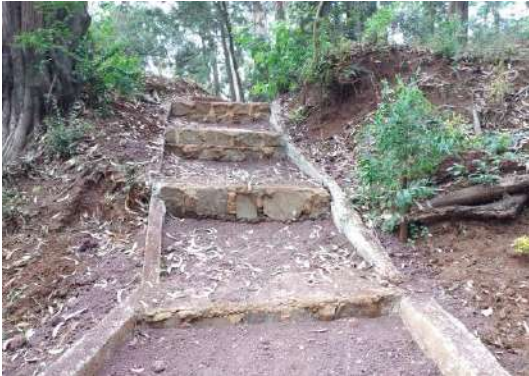
Figure 4.79: Uneven red ash stair
