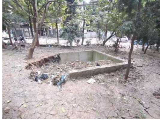
Figure 4.58: Uncovered manholes in the park compound
