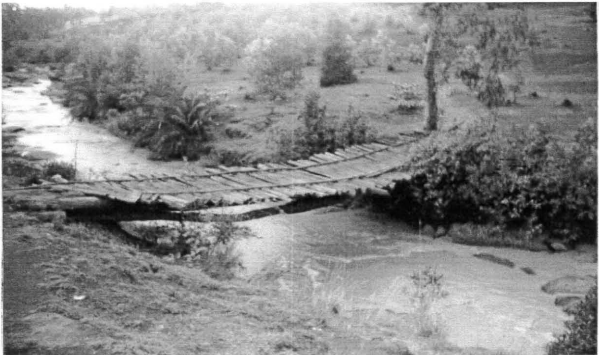
A bridge in the Yesemie jefore of the Girarina Yefermazigbe PA constructed by an NGO with the collaboration community members mobilized through their different iddirs .
