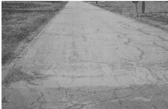
Figure 2.5 Block cracking pavement
