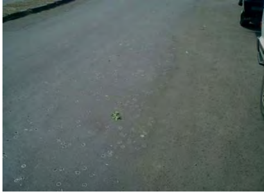
Figure 2.3 Alligator cracks imbedded
