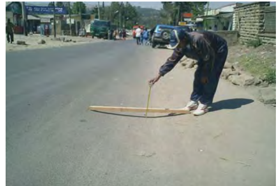
Figure 2.6 Sag in asphalt
