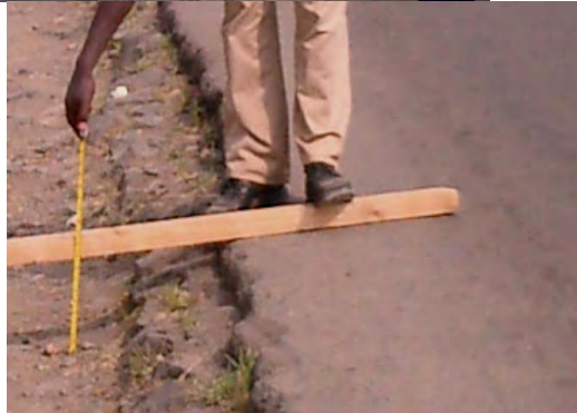
Figure 2.9 Edge cracking drop-off
