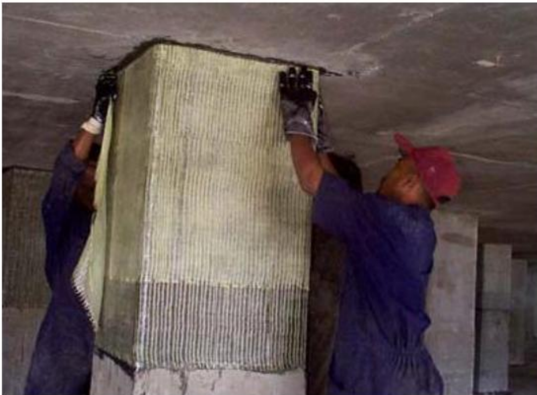
(b) Seismic retrofit of supporting columns for a cryogenic tank in Gujarat, India
