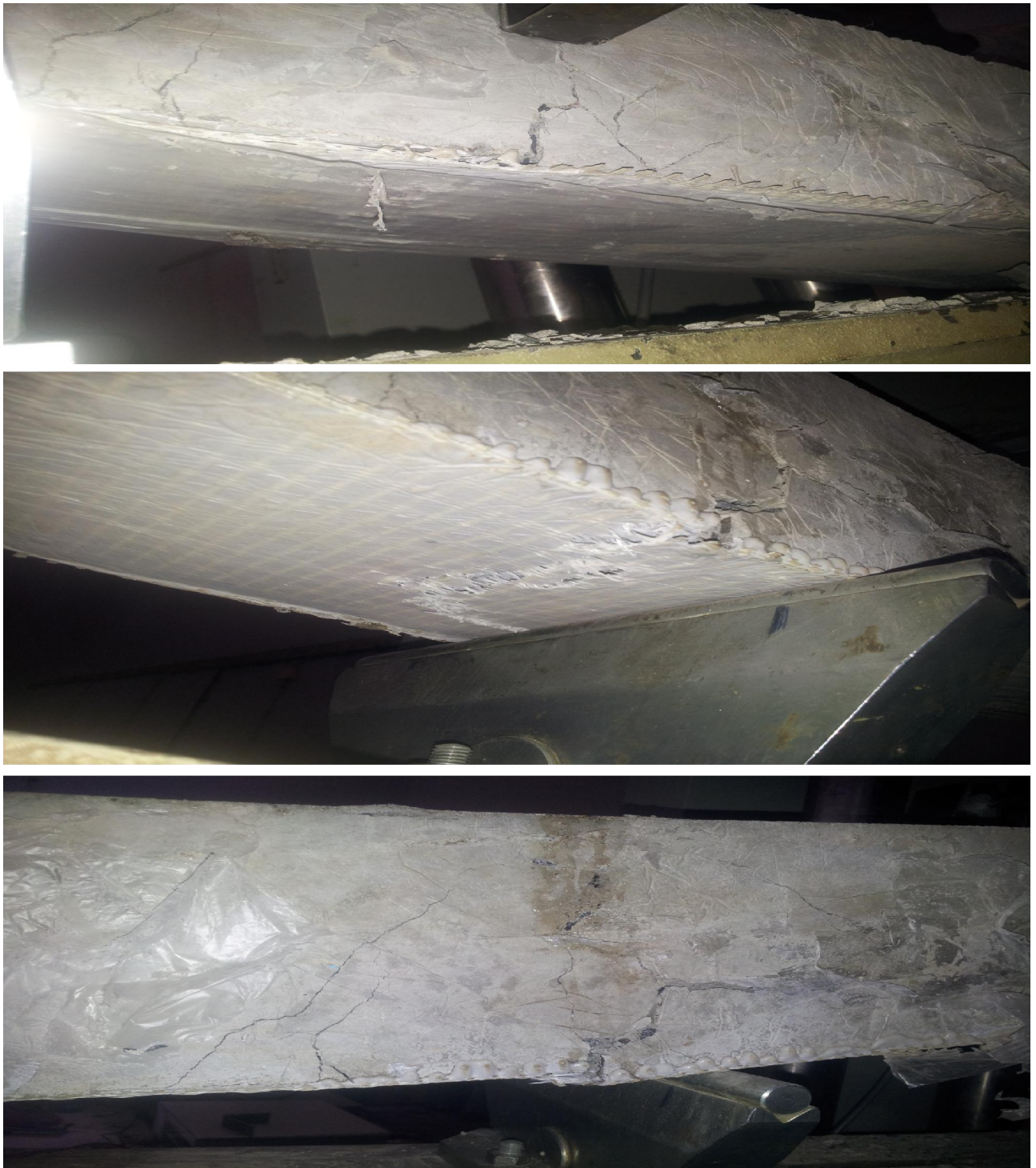
Figure 32 Flexural failures in group RF1, RF2 and RF3
