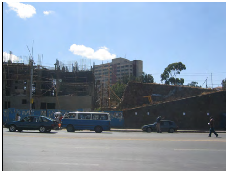
Fig.25. New construction at the eastern part of Meskel square where one of the two public toilets of the square used to be found.
