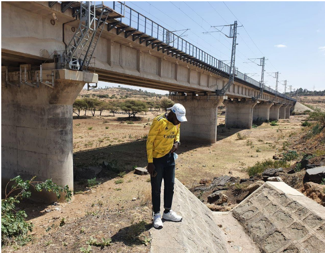
Figure 4.17: Railway bridge piers snapped during site-visitation
