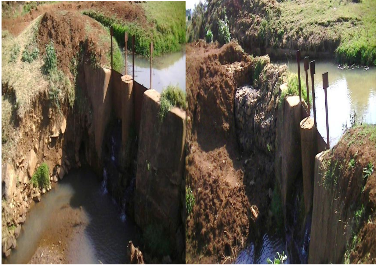
Figure 18: Poorly constructed irrigation canal in Yewla Kebele with landslide problem (Photo by the researcher, 2014
