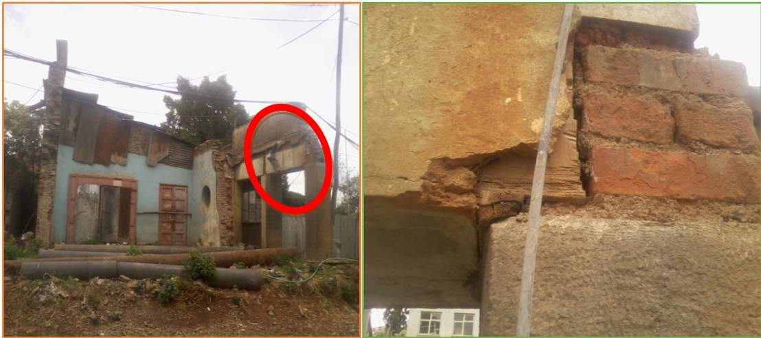
Figure 3: Loosely supported connection of timber beam with stone column
