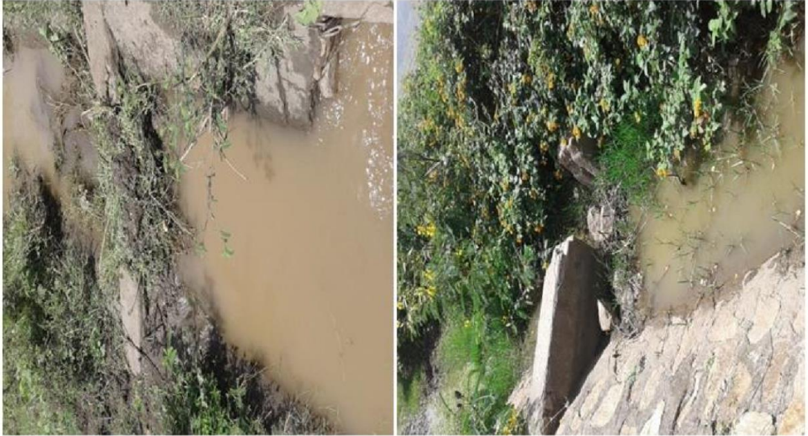
Appendix figure 7. 2: Un-functional drop structure
